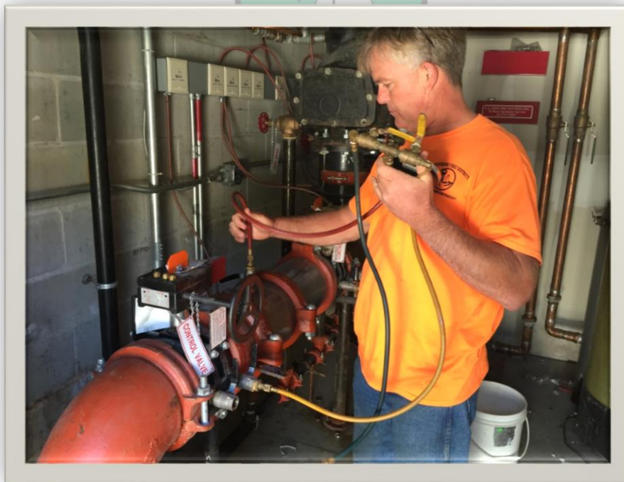
Picture 4: District Performing a Backflow Test
