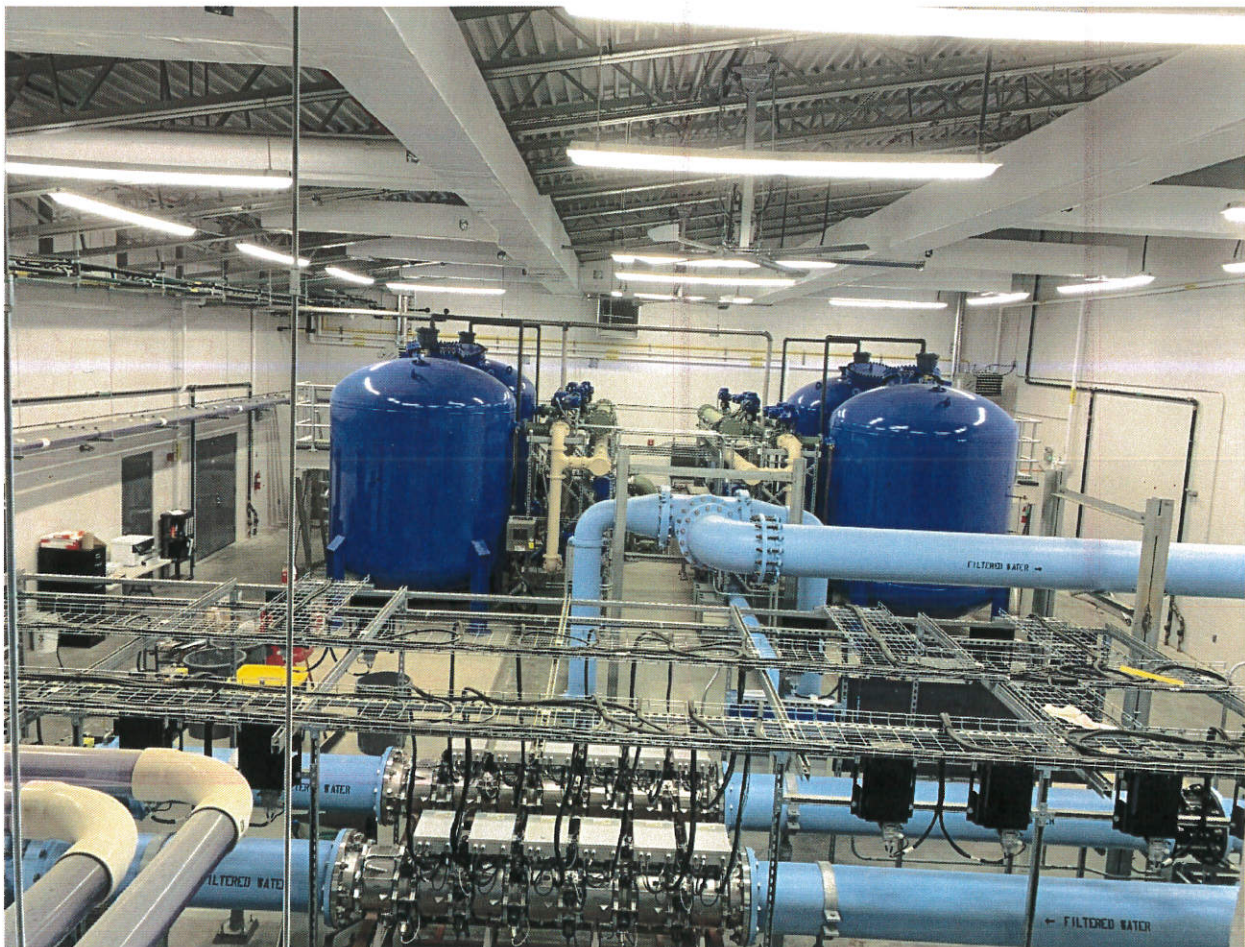
Picture 2: Maple Springs Water Purification Plant Filtration and Disinfection System
