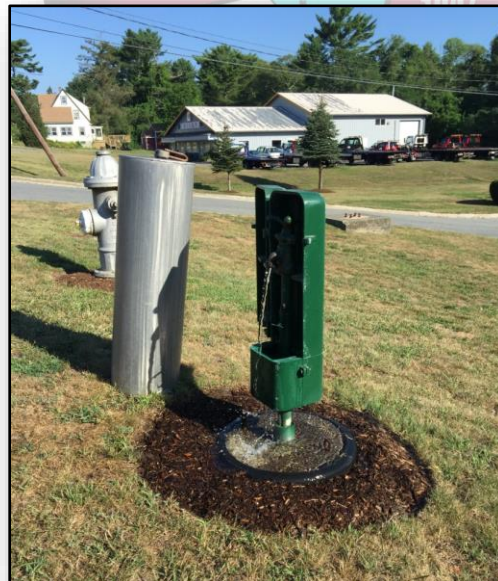
Picture 2: Secure Sampling Station in the Distribution System
