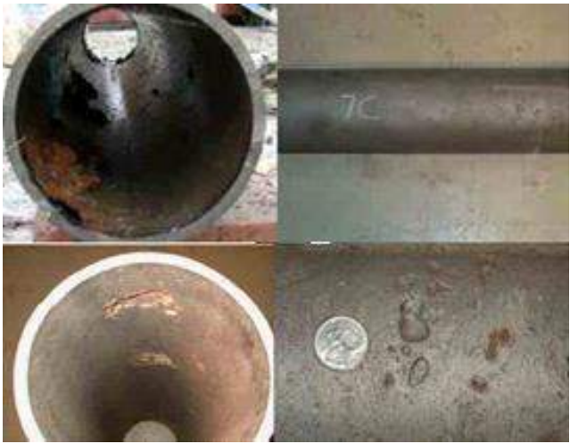
6" CI pipe with 10% measured loss
