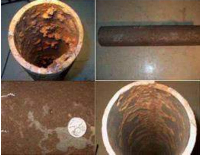
6" CI pipe with 4.2% measured loss
