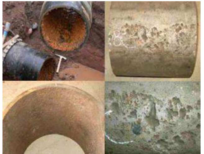
18" CI pipe with 18.5% measured loss
