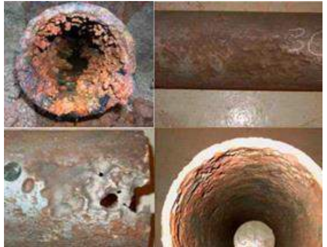
6" CI pipe with 47% measured loss
